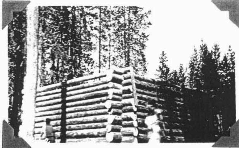
Start of construction of National Creek Snowshoe Cabin, Third Enrollment Period August 19th, 1934
