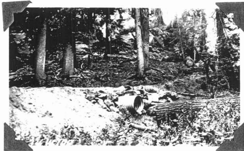
Culvert along Watchman-Castle Creek Loop Truck Trail installed with CCC Enrollees from Camp Annie Spring under supervision of Foreman Fred C. Patton Annie Spring Project No.4
