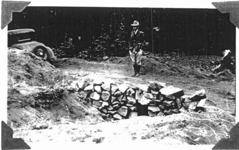
Culvert along Union Peak Loop Truck Trail installed with CCC Enrollees from Camp Annie Spring under supervision of Foreman E.L. Johns Annie Spring Project No.4 September 15th, 1934
