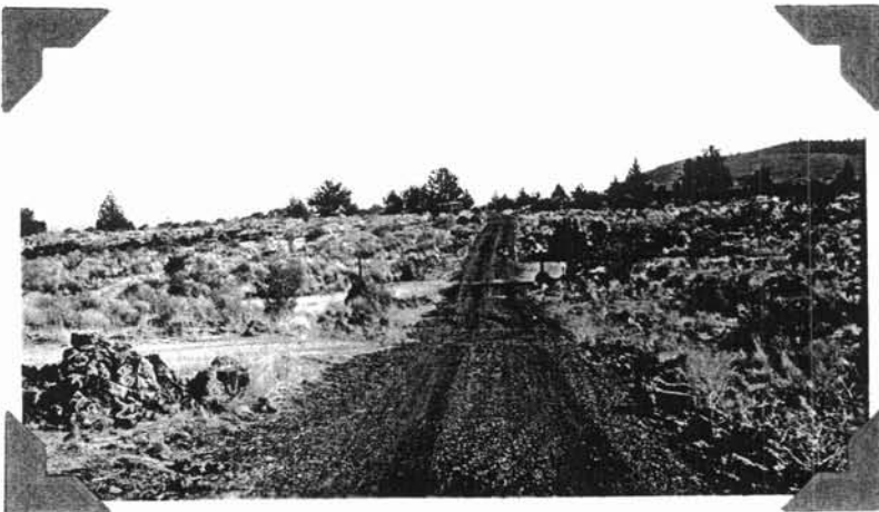
VIEWS OF ROAD BUILT WITH NIRA FORCES DURING THE WINTER OF 1933 - 34 LAVA BEDS NATIONAL MONUMENT
